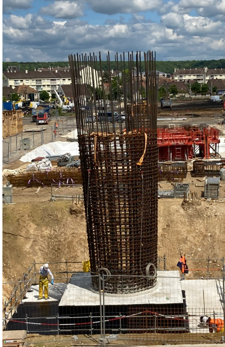
Top left: Aerial view of the structure bottom left: Interior view of the RaPL deck structure right: Reinforcement of the footing and shaft of Pile P4
